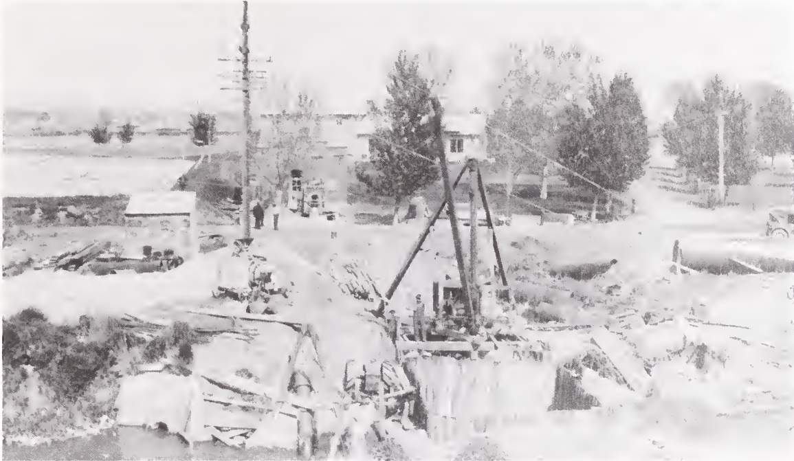
The east approach to the Bell Street Bridge under construction (Ruth Torrence).
